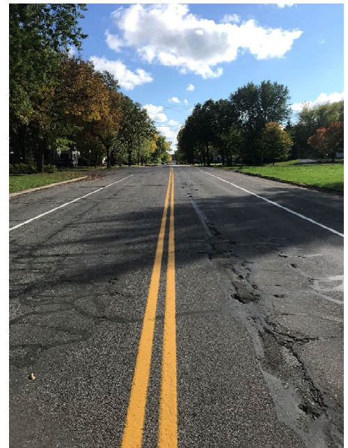
Existing pavement condition south of Maple Ave
