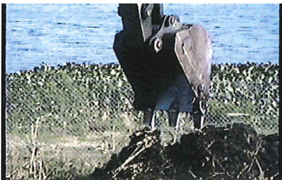
Bucket Teeth are spaced 6 to 8 inches apart Note the sludge is not sticking to the bucket
