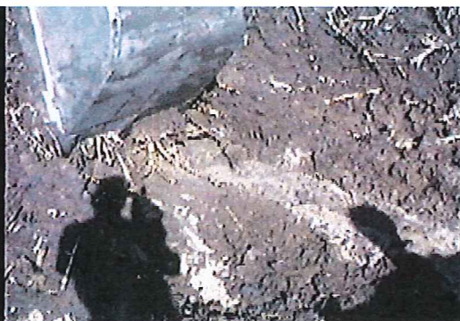
Stop digging when you see sand layer Note the root growth in sludge layer
